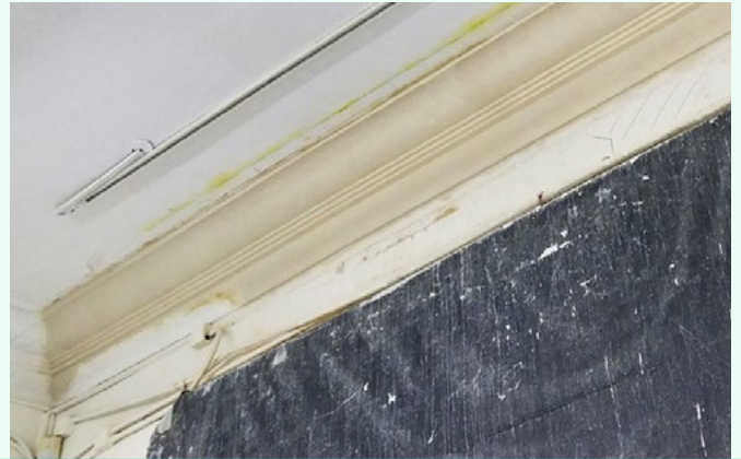
▼ 修理好的簷口裝飾橫帶等待上漆。 A finished cornice repair prior to painting.
