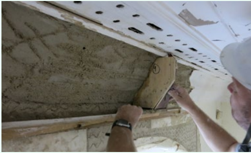
▲ 資深技師先將木尺固定在牆上，然後把模板(俗稱「馬仔」)架在木尺上，再以木尺作軌道，運行模板在底層石膏上，刮出簷口的雛形。此修復技巧乃110年前建造簷口裝飾的同一方法。 Experienced craftsman running the plaster base of the cornice using a 'horse' which is guided by a 'running rule' fixed to the wall. The cornices are repaired in the way that they were originally constructed 110 years ago.
